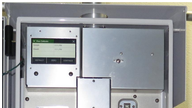
Figure 6-10 Flow System Cover Removed
